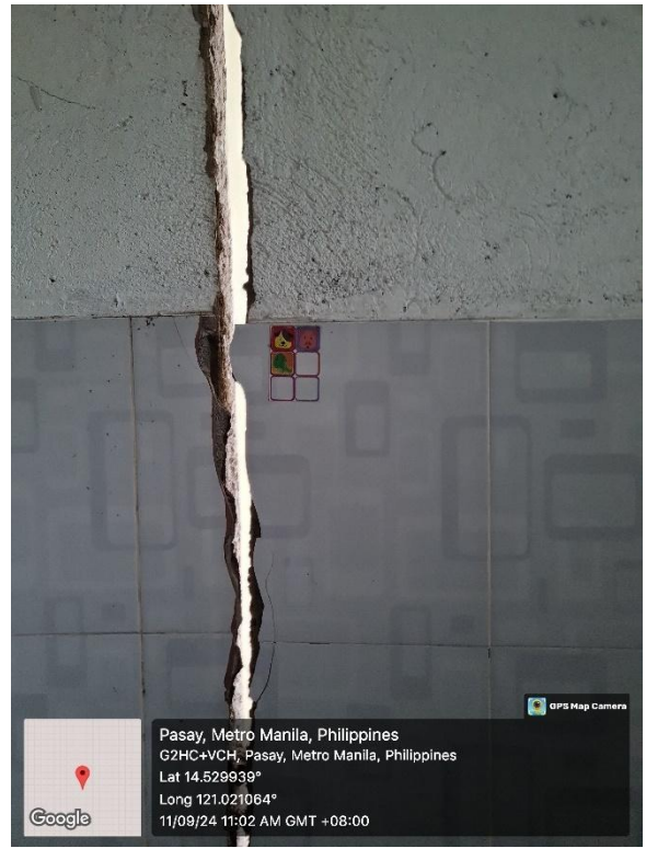
Crack in one of the toilet rooms
