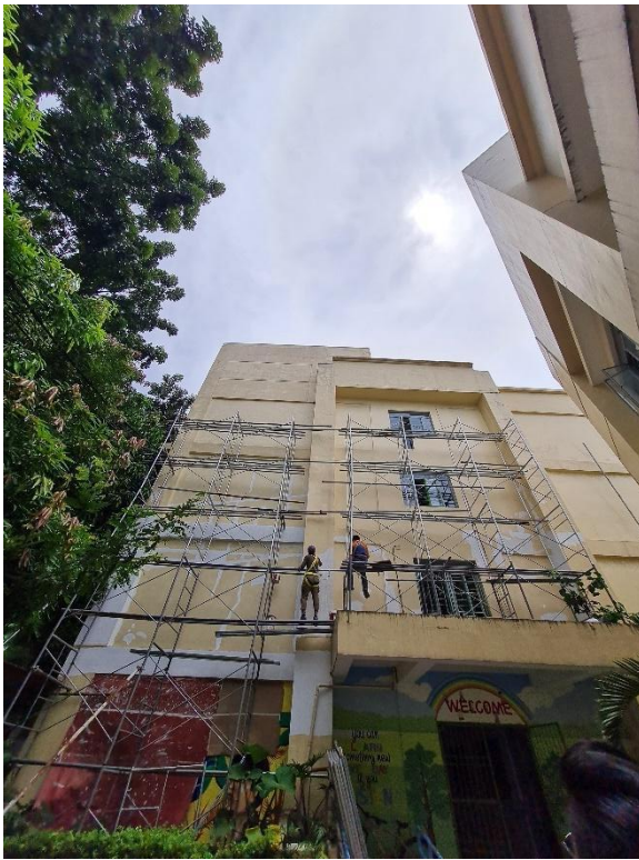
There is an ongoing renovation to the affected building at the time of visit.
