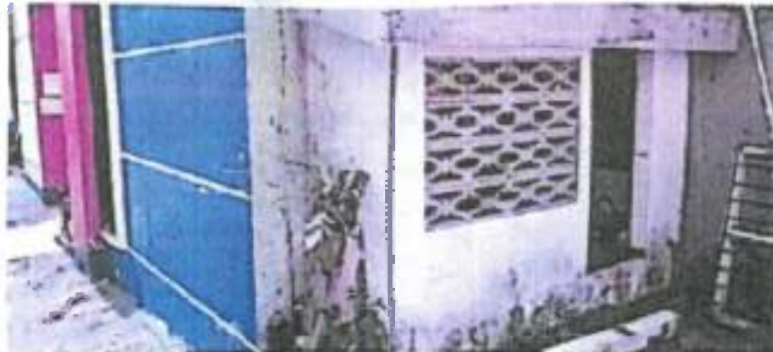
WATER PUMP, PRESSURE TANK & GENERATOR ROOM
